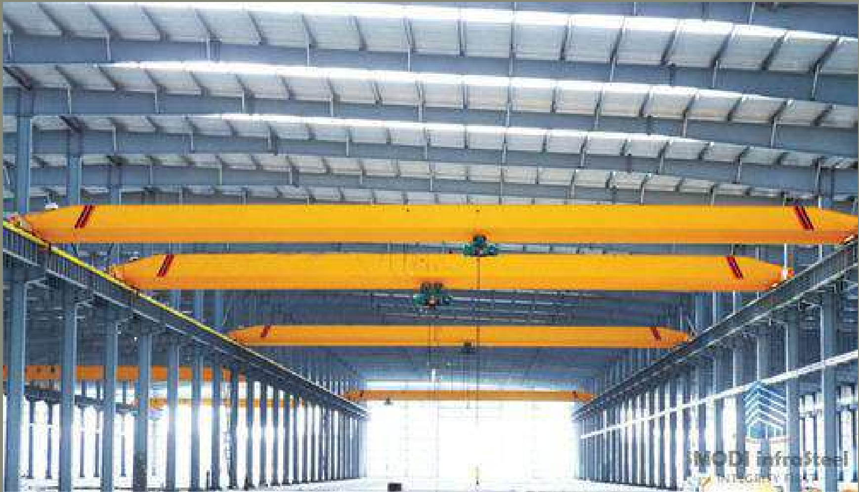
PEB with EOT crane
